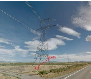
< 500 KV DC Transmission Lines and Tower
