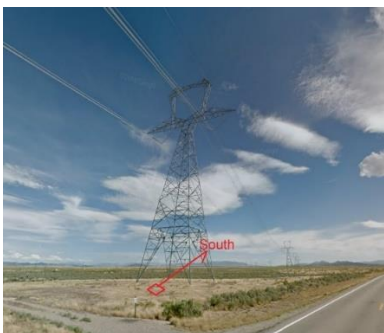
< 500 KV DC Transmission Lines and Tower
