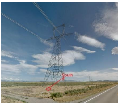
< 500 KV DC Transmission Lines and Tower
