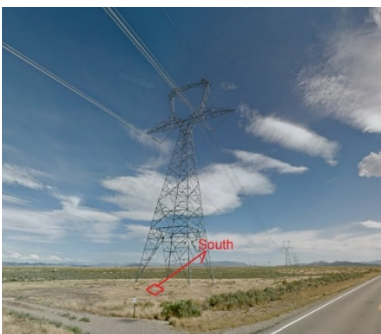
< 500 KV DC Transmission Lines and Tower
